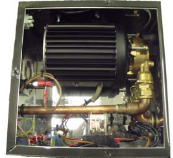
Pump Motor Compartment
